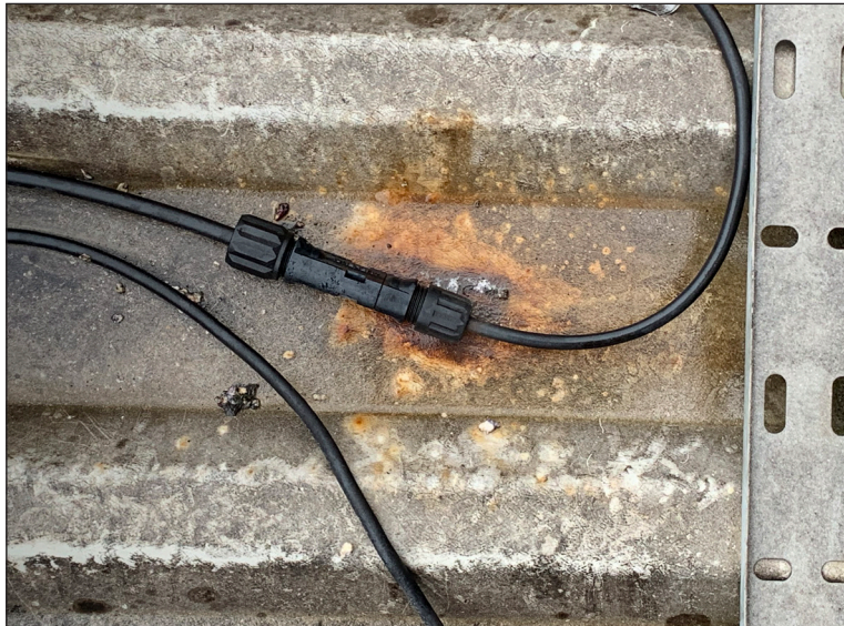
Figure A6.4 DC connector leakage. Discoloration of roof caused by leakage current, due to mis-matching connectors. (Reproduced by kind permission of Helios Solar O&M)
