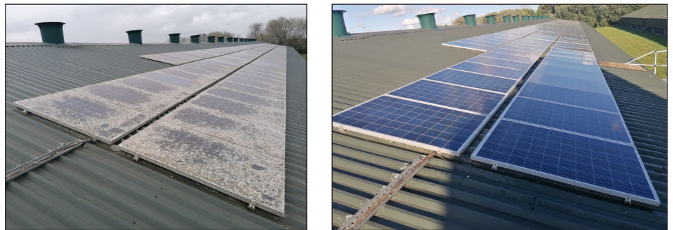
Figure A6.2 Solar panels before and after cleaning. Shading of solar panels due to foreign matter can lead to overheating. (Reproduced by kind permission of Helios Solar O&M)
