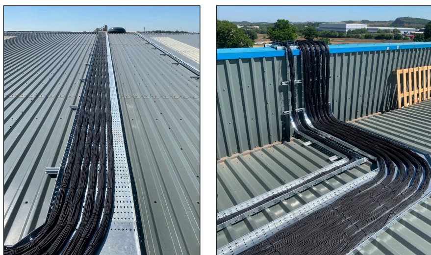
Figure 5.5.3 (left) String cables in tray prior to final cover plate and (right) cable management over parapet wall prior to final cover plate (Reproduced by kind permission of Chris Roberts, Clean Energy Consulting Ltd)
